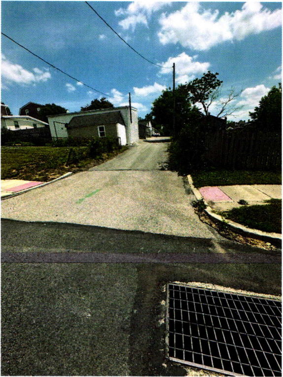
Exhibit C: Downward slope of alley
